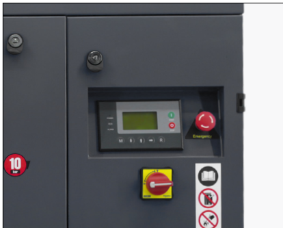
Emergency Stop and control panel
